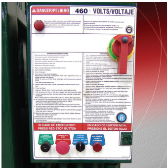
Standard controls: Key Lock On/Off Auto Cycle, Emergency Stop, and Platen Raise/Lower. Baler Ready light indicates the unit is operational. Shown with optional "Bale Made" light and electrical disconnect.
