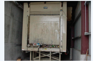
The BlokPak 3000 fits nicely into existing transfer stations with over-the-top feed systems such as this one located in Black Foot, ID.
