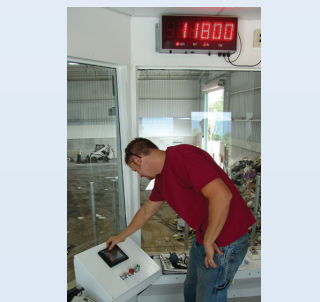
The BlokPak 3000 control station features a color touch-screen interface. This installation also has an integrated weighing system that displays the accumulating weight on-screen and on overhead monitors while the waste is being processed.
